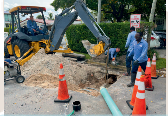
Randy Stokes, Public Works Director operating the combination load assisting the Utilities Division replace a sewer line connection on Biscaya Drive. Pictured: Randy Stokes, Wayne Taylor, Utilities Supervisor Kenny Chaviano and Curtan Turner.
