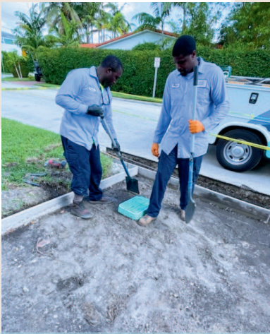
Wayne Taylor and Curtan Turner installing a water box for a Resident.
