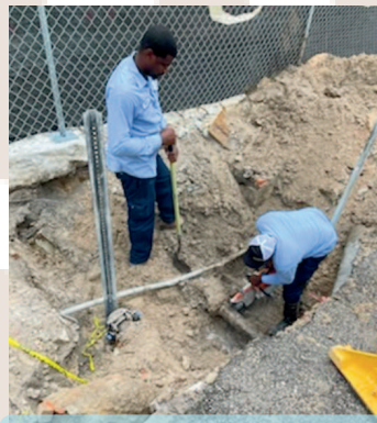
Wayne Taylor and Curtan Turner from the Utilities Division capping a waterline.
