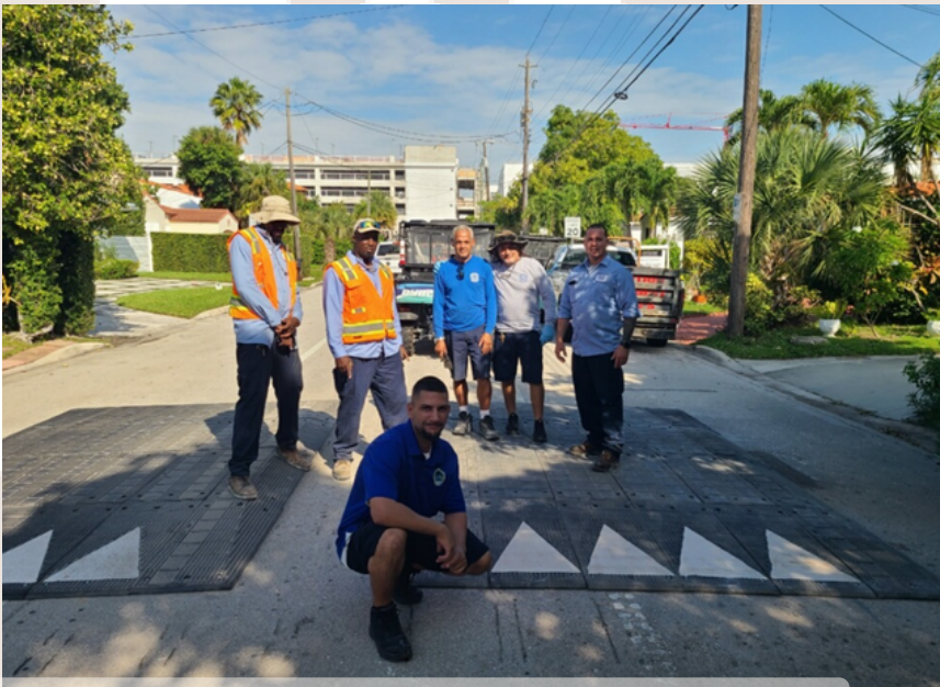
The Utilities Division and Maintenance Division worked together to install traffic-calming speed tables on Byron Ave.
