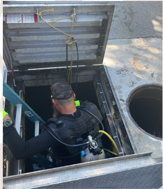
Public Works Operations Manager Felix Alvarez performing underwater repairs at the 94th Street Pump Station
