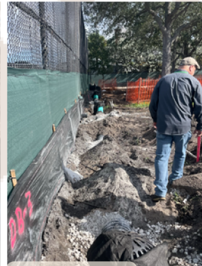
Public Works Director Randy Stokes performing a drainage Inspection at the 96th Street Park Project.
