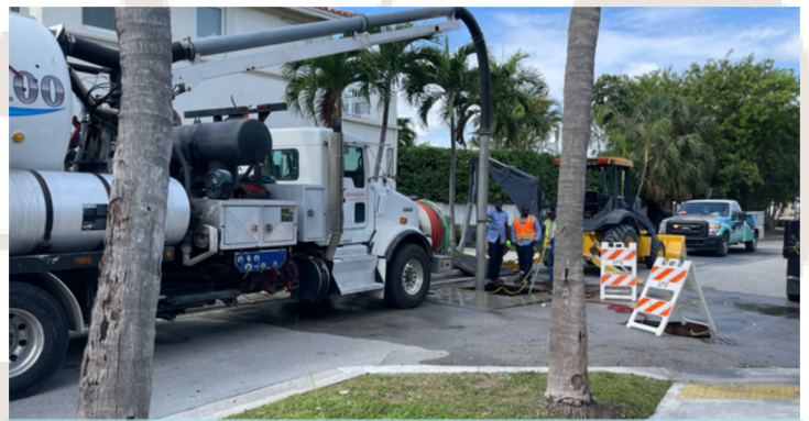
Water & Sewer Maintenance Workers Wayne Taylor and Curtan Turner supervising Vactor truck activities at the 94th Street Pump Station.
