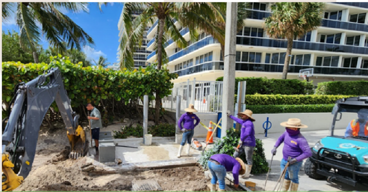
Water & Sewer Supervisor Kenny Chaviano operates the combination back loader and Maintenance Supervisor Josvani Iglesias guides excavation efforts at the 96th Street Beach End Shower.
