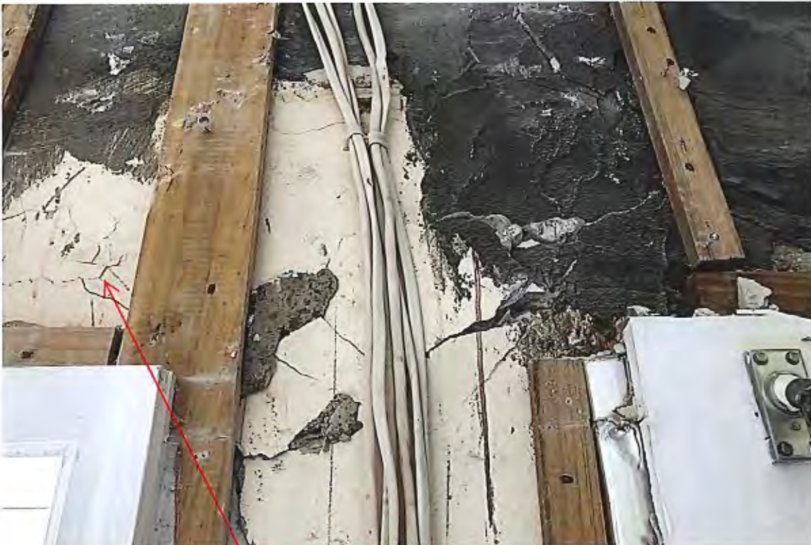
CRACKS IN TIE BEAMS AND TIE COLUMN
