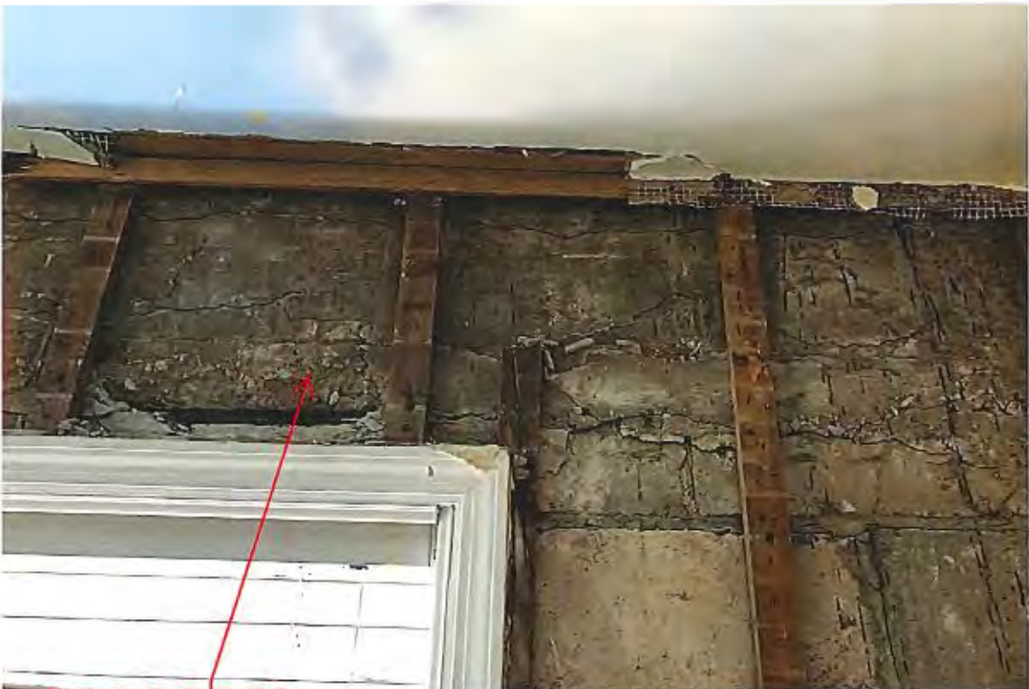
EXTENSIVE SPALLING IN TIE BEAM
