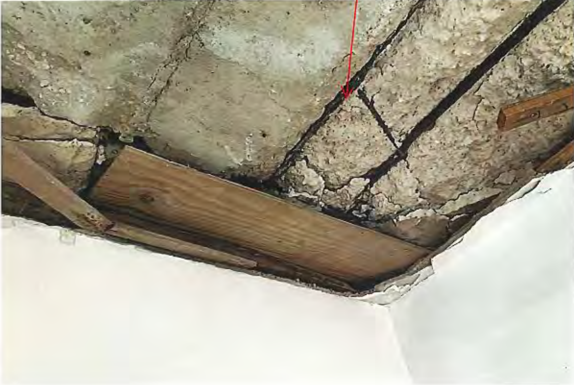
EXTENSIVE DAMAGE IN CONCRETE BEAM
