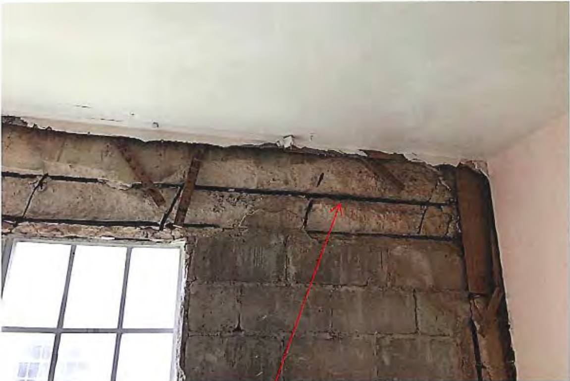
TOTALLY EXPOSED REINFORCEMENT
