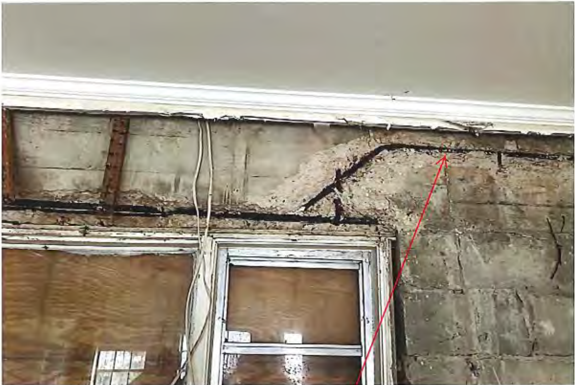
DAMAGE IN TIE BEAMS
