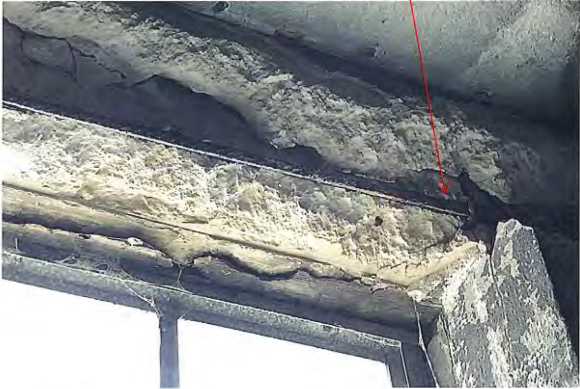
FALLEN CONCRETE AND EXPOSED RUSTED REBAR
