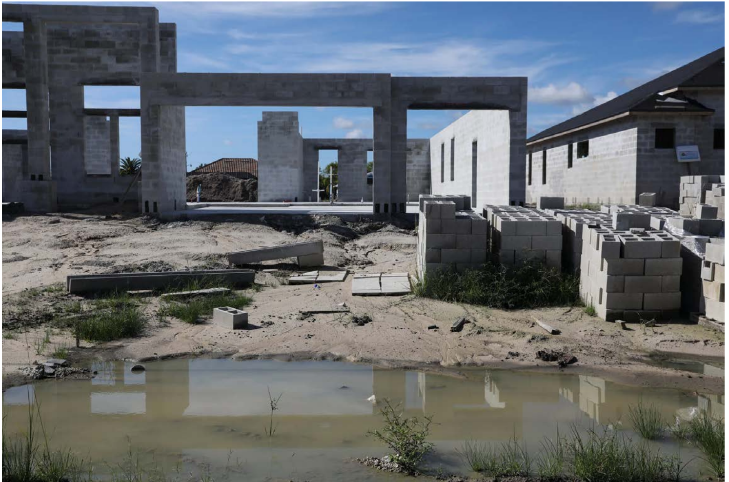
A house under construction in South Gulf Cove, Fla., a town ninety minutes south of Tampa on Gasparilla Sound. Eve Edelheit for The New York Times
