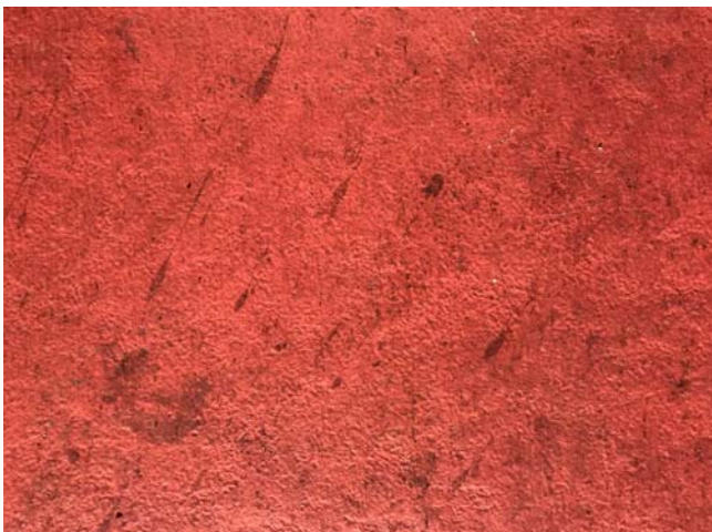
Picture C – “Sidewalk with 6 Coats of Staining”
