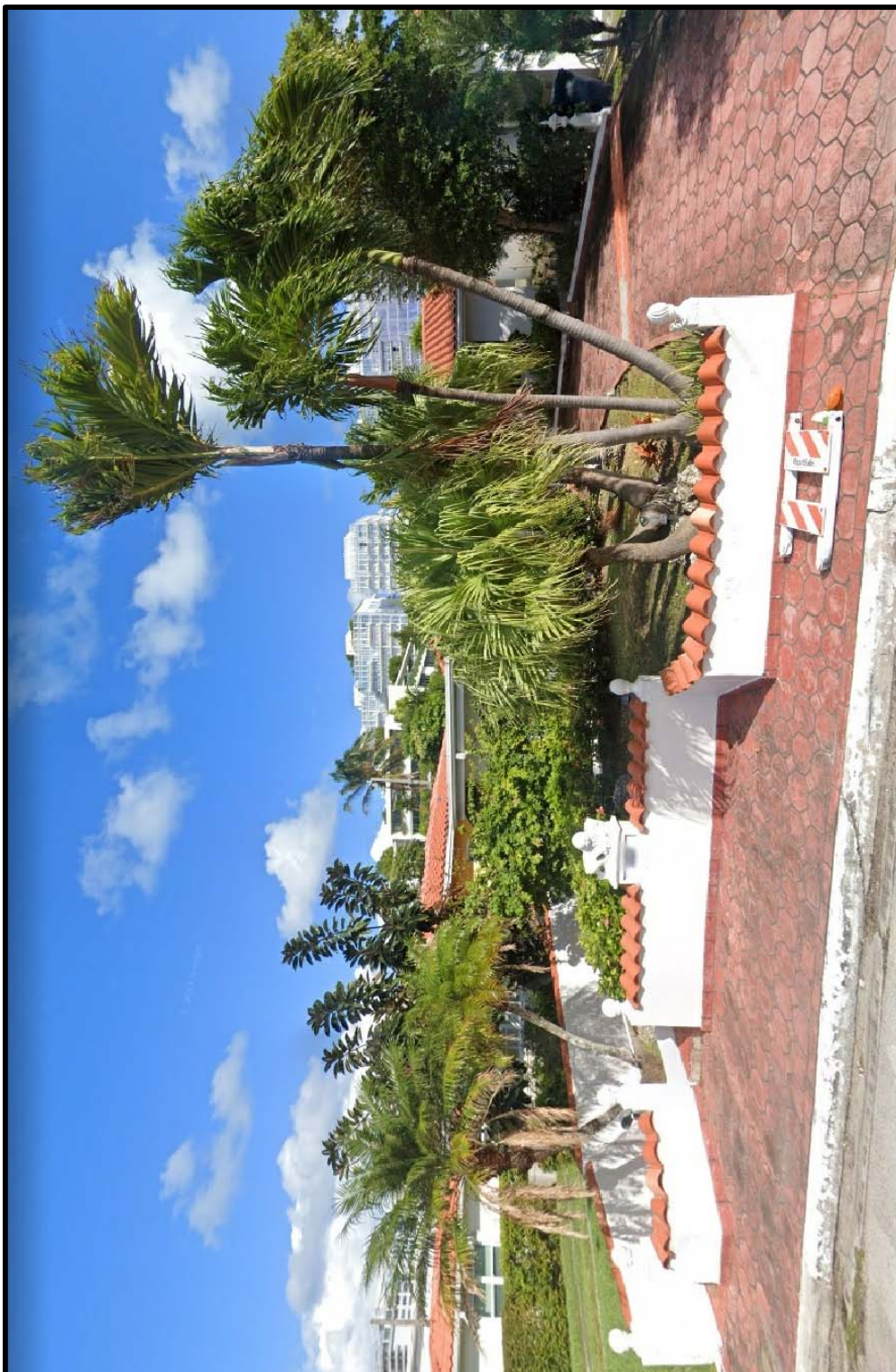
EXISTING FRONTAGE (ALL HARDSCAPE TO BE DEMO - NON COMPLIANT IN ROW.)
